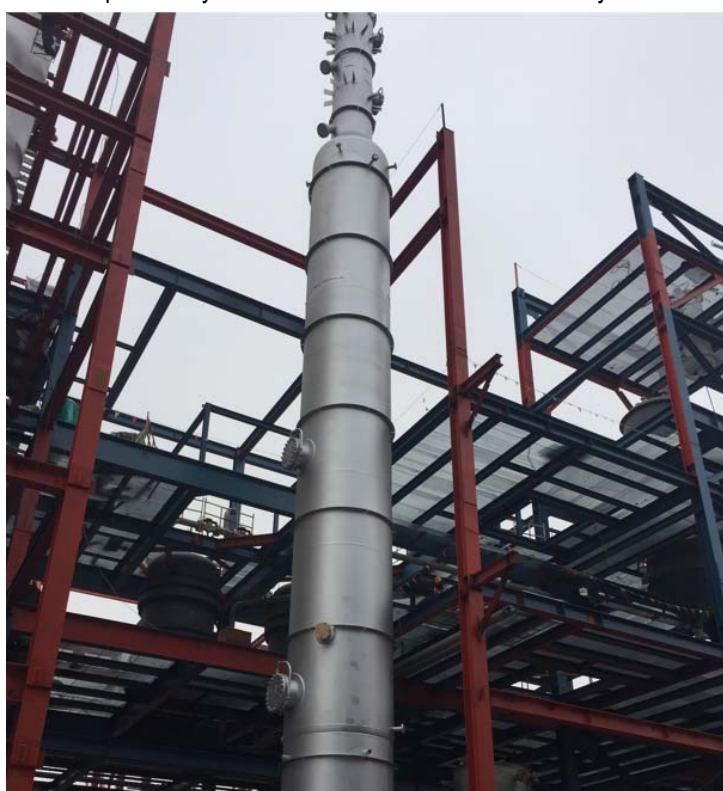
Fig. 2: Detail of Ammonia Absorber - XLX Euromel® Melamine Plant, Xinjiang, China – World's largest single-train HP melamine plant, 60,000 MTPY, operating since 2016
