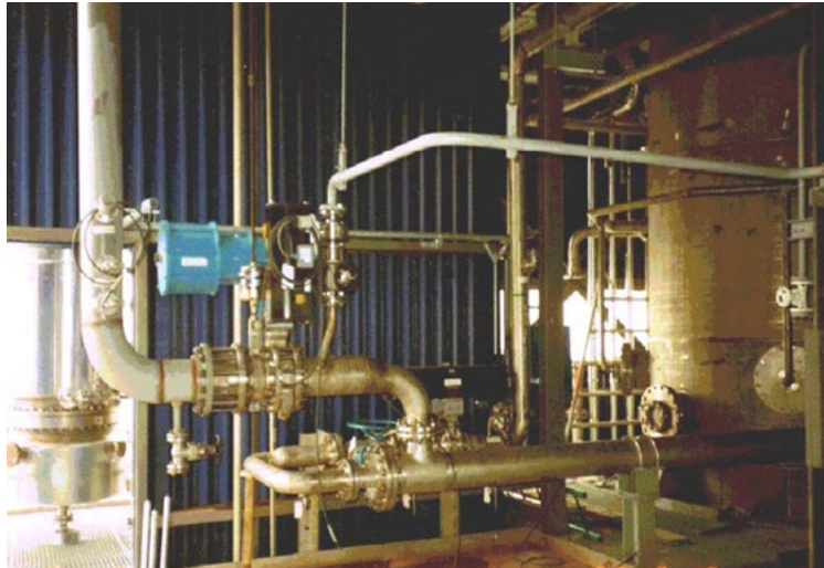
Figure 2: Grande Paroisse Pipe Reactor at DSM Geleen (now OCI)
