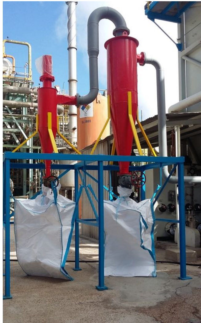
Figure 1. Main and secondary cyclone filters. Ejector not shown. for ejector see figure 2.
