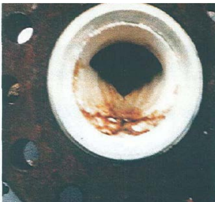
Figure 5: Clogged outlet line of a ammonium carbamate safety valve
