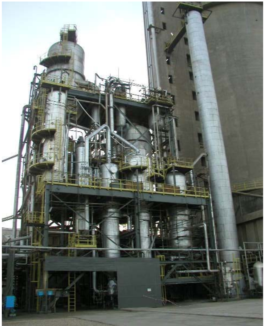
Picture 1: Snamprogetti Medium Pressure Recirculation section
