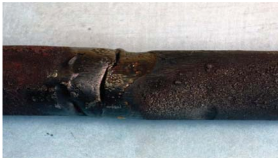
Figure 8 - Case 13: Erosion corrosion of preheater tubes near support plates. Coarse crystalline magnetite was found ( R = 0.93 ) next to the erosion-corrosion place.
