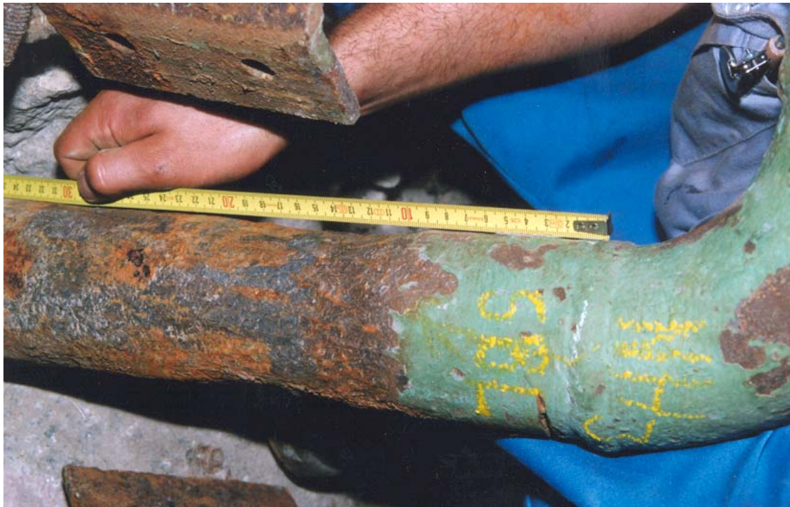
Photo 4: Severity of external corrosion at carbon steel ammonia pipeline
