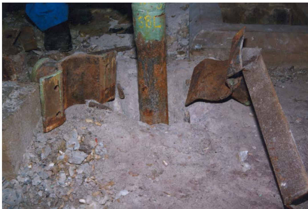
Photo 3: Crevice corrosion at carbon steel ammonia spill back line
